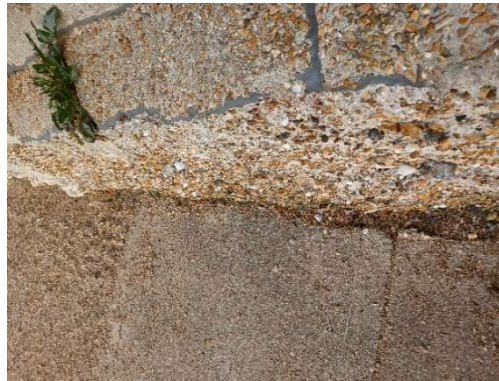
Plate 1: Spalling of concrete on seawall
